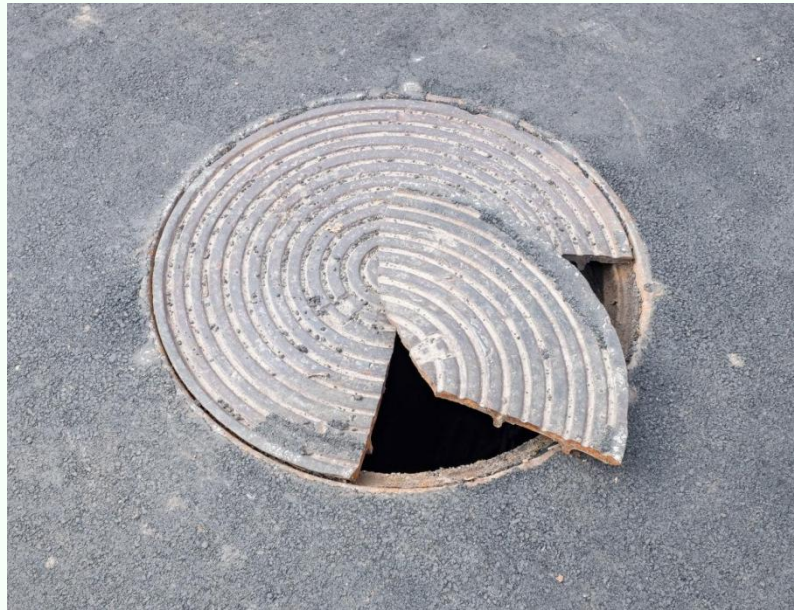
Figure 1. A cast iron sewer cover broken as a result of external impact.
